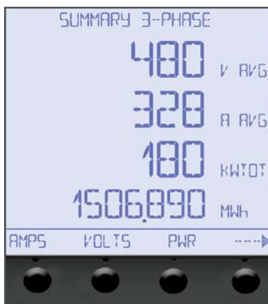
Front panel display showing function selection buttons and 3-phase voltage, current and power summary display.
